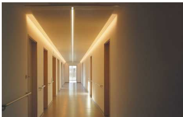
ceiling mounted light in the hallway of a retirement home 200105
