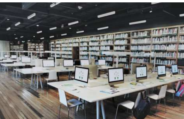
Pendant luminaire above workstations in the library with indirect RGB+WW lighting 200112
