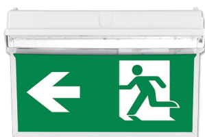
LED emergency light/escape route luminaires
